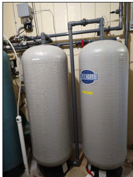
Well pressure tank
