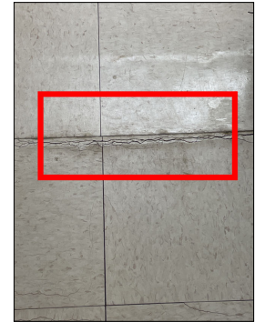
Damaged flooring noted
