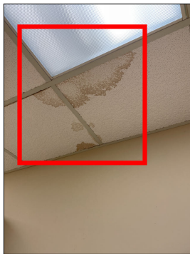
Evidence of past moisture damage noted
