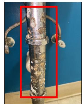
Corrosion on pipes
