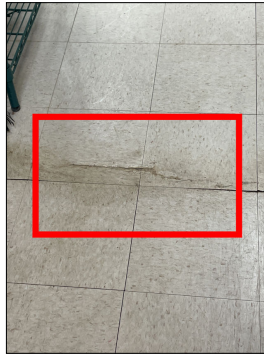
Damaged flooring noted
