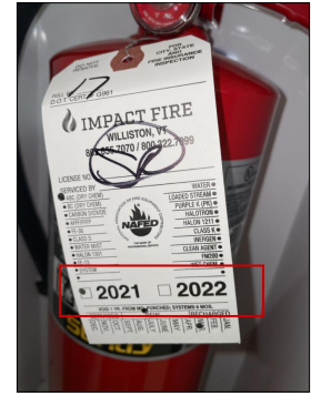
Fire extinguisher not properly tagged
