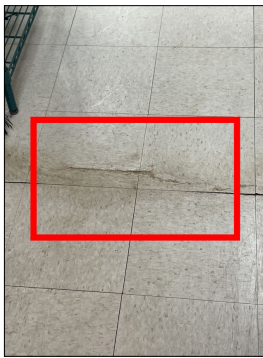
Damaged flooring noted
