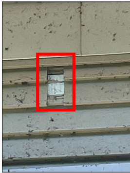
Gaps in vinyl siding
