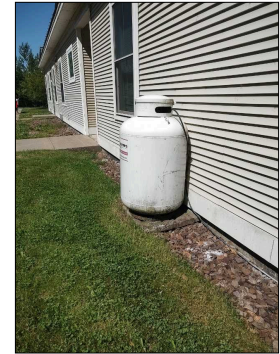
LP gas tank location
