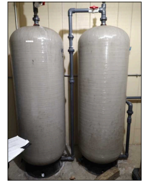
Well pressure tank
