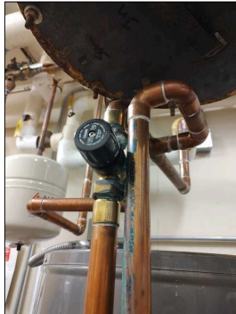
Thermostatic mixing valve for the hot water heater
