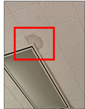
Water stains: dry
