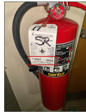
Fire extinguisher not properly tagged
