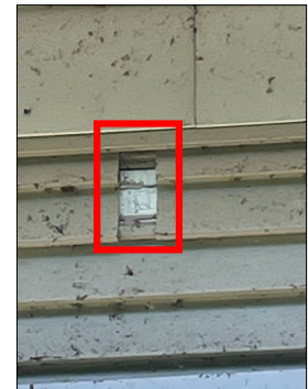
Gaps in vinyl siding
