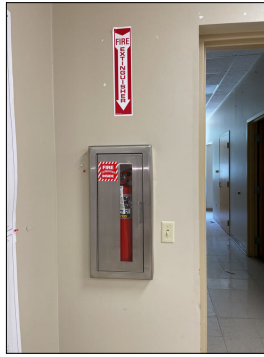
Fire extinguisher mounted
