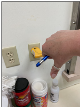
Receptacle that needs to be GFCI protected
