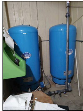
Well pressure tank
