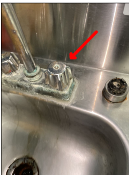
No water from cold side of faucet
