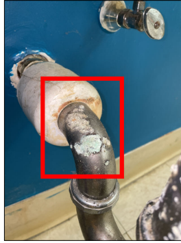
Corrosion on pipes
