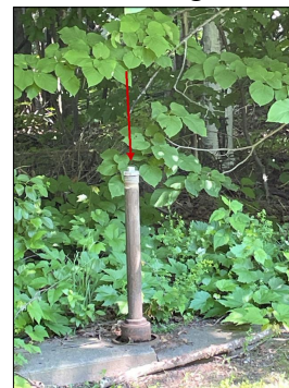
Oil fill pipe location
