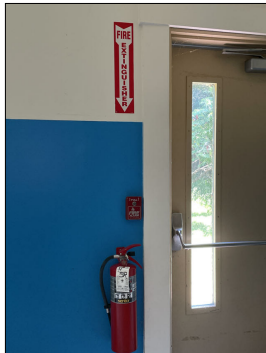
Fire extinguisher and marking
