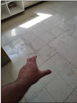
Evidence of vapor diffusion and capillary suction: moisture affecting the flooring
