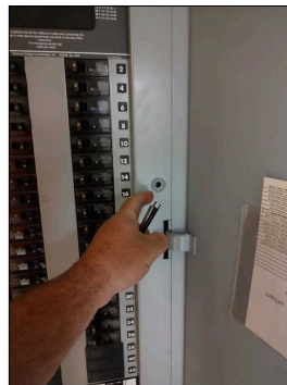
Missing panel box screw noted
