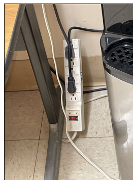
Extension cord being used for permanent power
