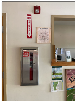
Fire extinguisher mounted
