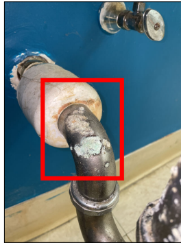
Corrosion on pipes
