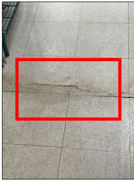
Damaged flooring noted
