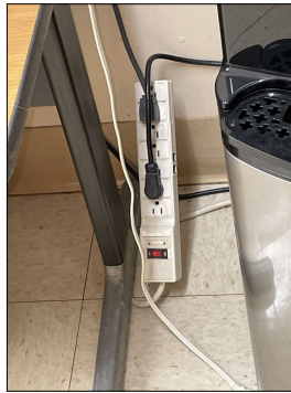
Extension cord being used for permanent power
