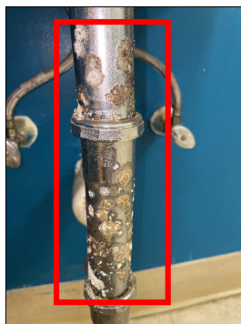
Corrosion on pipes
