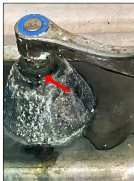
Water faucet leaking
