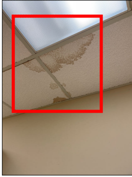
Evidence of past moisture damage noted
