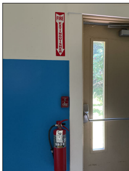
Fire extinguisher and marking
