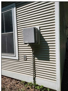
Septic tank alarm
