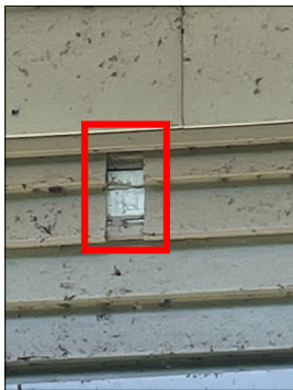
Gaps in vinyl siding
