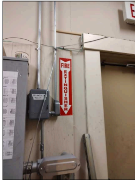
Fire extinguisher marking
