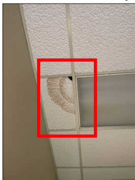
Water stains: dry
