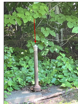
Oil fill pipe location
