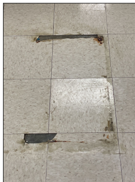
Damaged flooring noted
