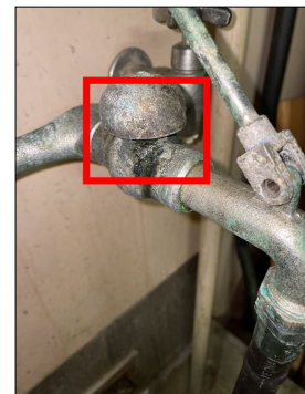
Water faucet leaking at the base
