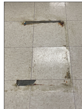
Damaged flooring noted
