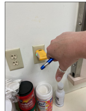
Receptacle that needs to be GFCI protected
