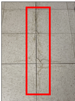
Damaged flooring noted
