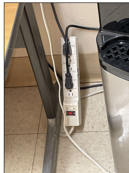
Extension cord being used for permanent power
