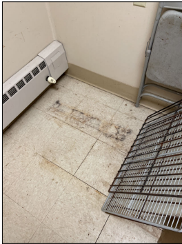
Damaged flooring noted
