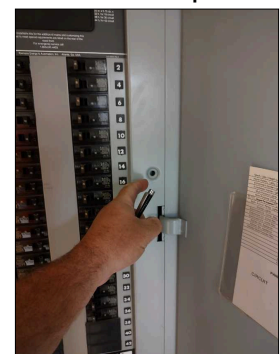
Missing panel box screw noted
