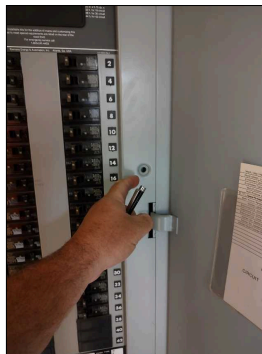
Missing panel box screw noted
