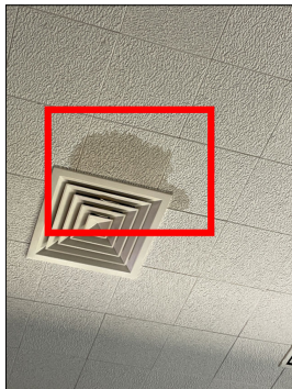
Water stains: dry
