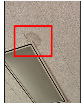
Water stains: dry
