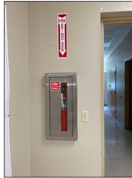
Fire extinguisher mounted
