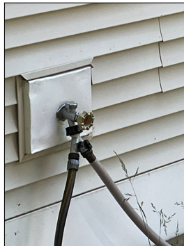
Front exterior faucet
