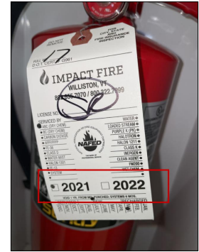
Fire extinguisher not properly tagged
