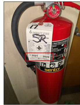
Fire extinguisher not properly tagged
