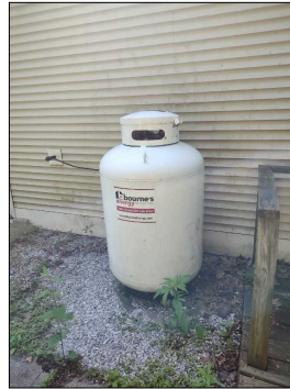
LP gas tank location
